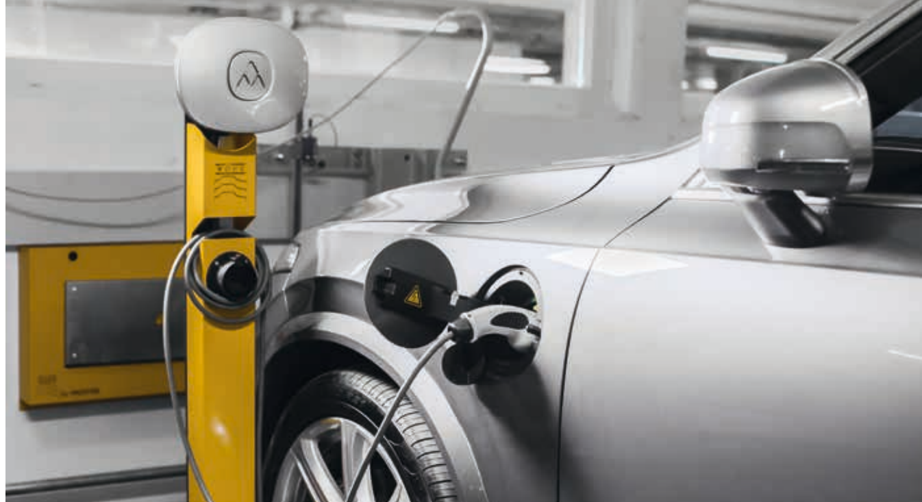
In the parking system the platforms are equipped with charging stations for electric cars, commonly used in Norway.
