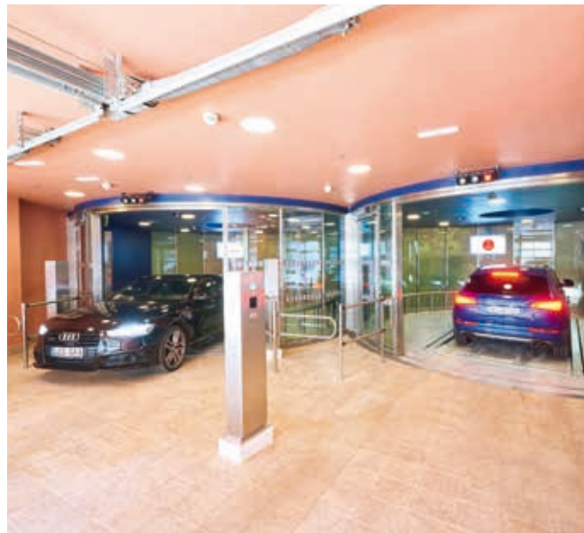
Two independent seven-storey Parksafe systems are located beneath the Palais.
