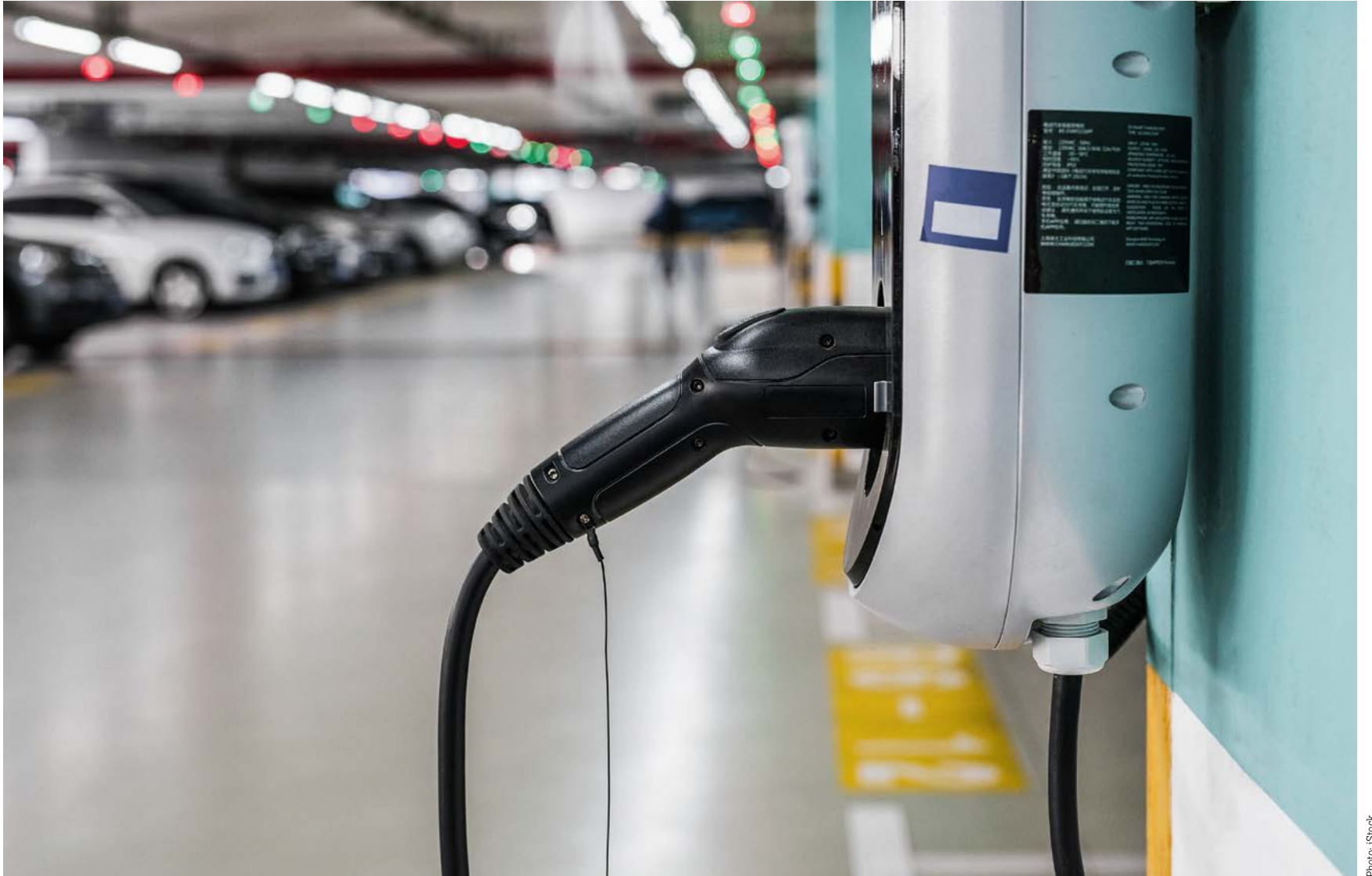
Multi-storey car park charging station
